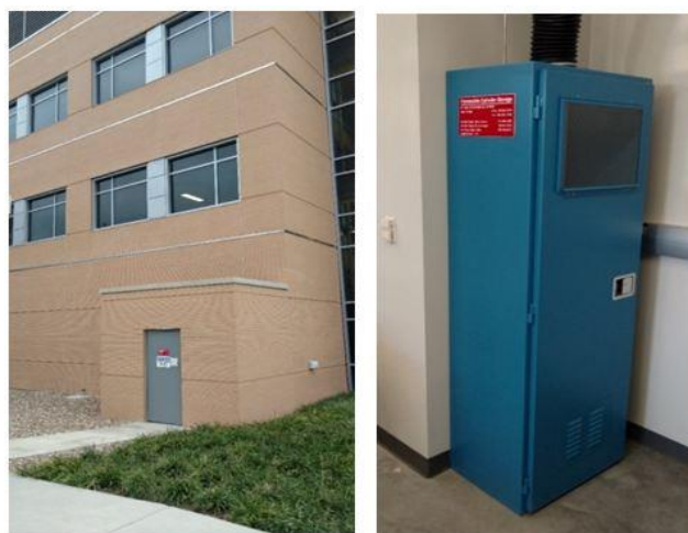
Figure 5: Left: Outdoor flammable gas storage building (7.5 ft × 12 ft) with open roof and concrete floor (note concrete sidewalk for wheeling cylinder carts). Gases are piped into the lab to distribution panels located at the ends of the ventilated enclosures and inside hoods. Right: Ventilated gas cabinet (Safety Equipment Corporation, 7000 series) designed for storing flammable and toxic gases located in the lab.
